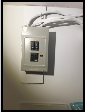
Sub Panel Neutral and ground wires must remain separate Electric code violation
